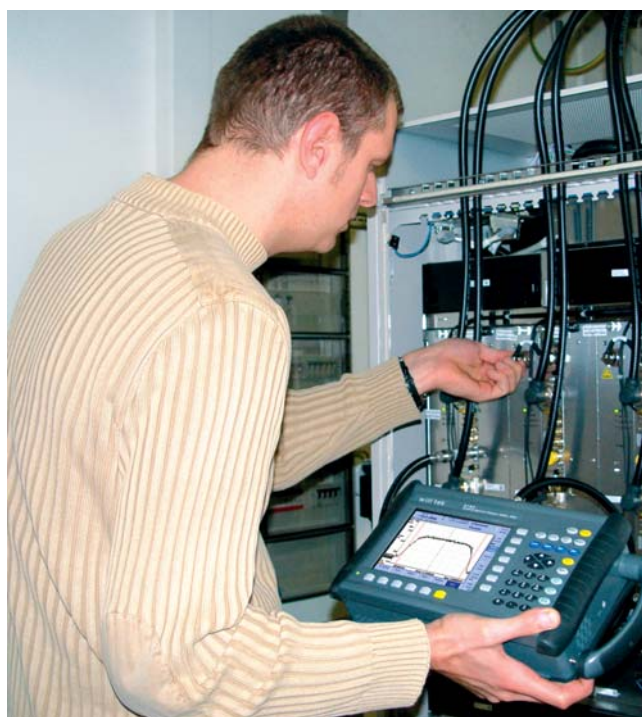
Channel power measurements at a UMTS Node B
